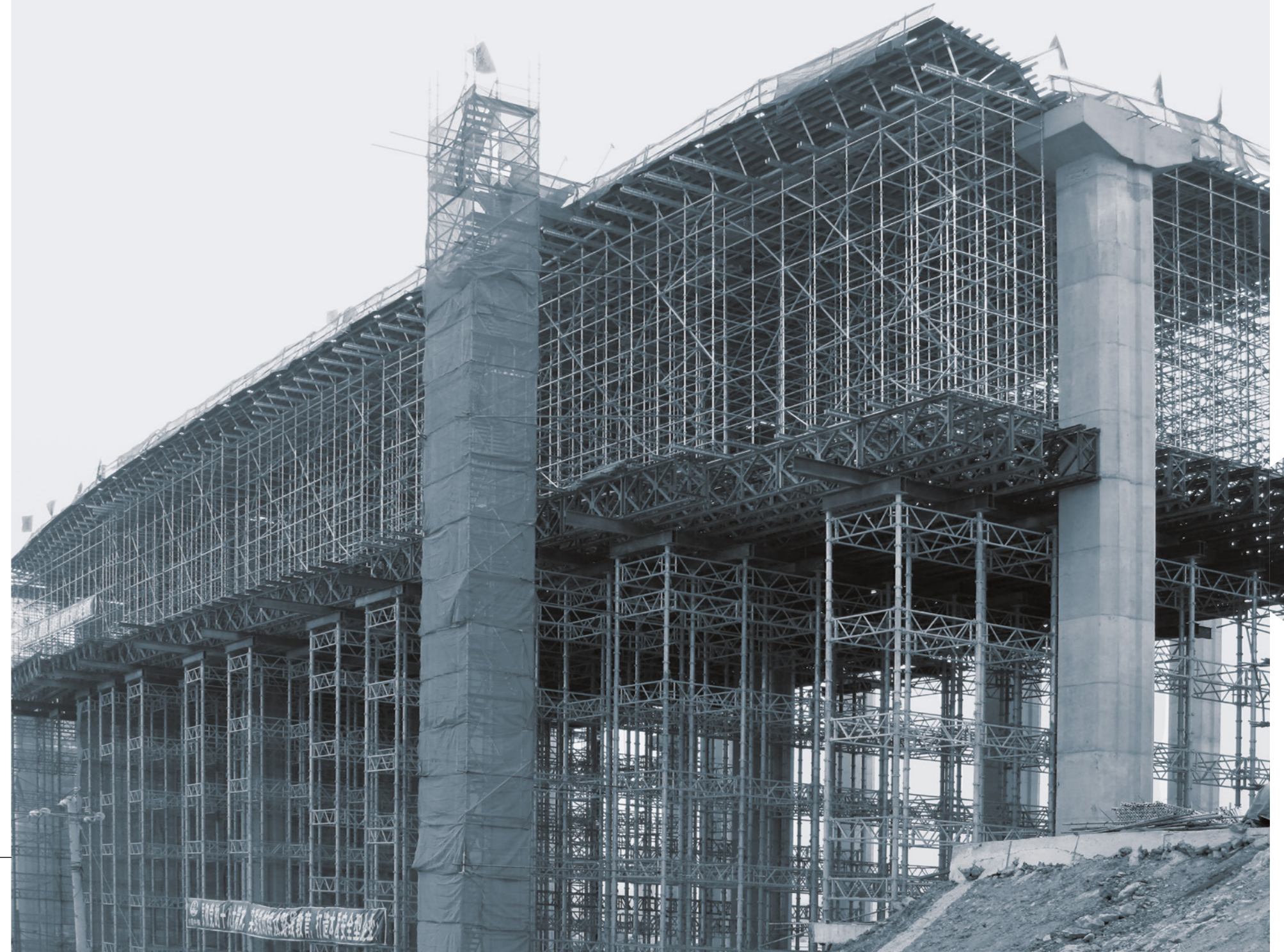
Guilong Highway in China. One million cubic metres of SPS, Duralok and SBS 135 material were used for the construction of the 12 km long Highway in the Guizhou Province. Special designs of shoring had to be done for the project.
