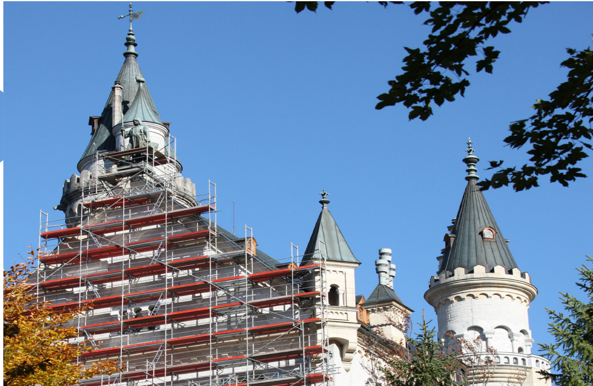
Castle Neuschwanstein in Germany. Narrow access roads, impassable terrain and crowds of visitors notwithstanding, Scafom-rux SUPER 65 scaffolding system in combination with a modular scaffolding system was erected to renovate the exterior façade of the globally known historic building.
