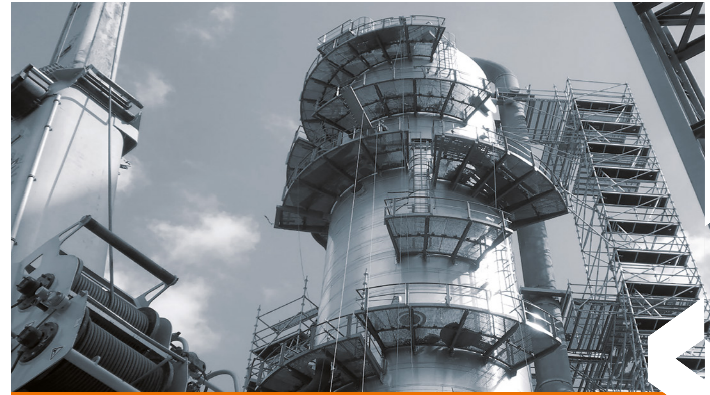
Europoort Power Plant in the Netherlands. The multidirectional RINGSKAFF system was ideal for the work on the power plant in Rotterdam. Thanks to its flexibility, the scaffolding could be adapted to the challenging shape of the object.
