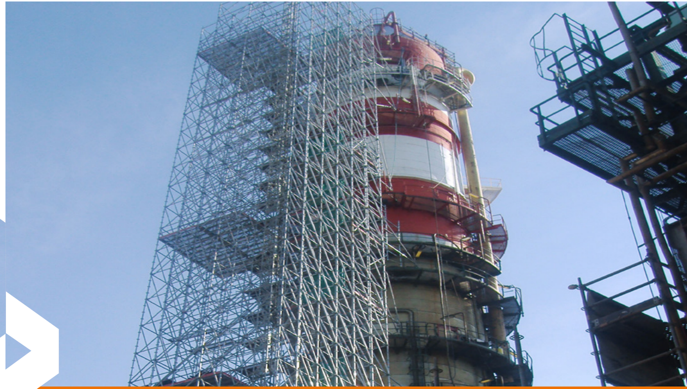
Repsol Refinery in Spain. The assembly of the 90 metres high RINGSCAFF scaffold for sandblasting work at the refinery in Tarragona was a real statical challenge. The difficulties posed by the temperature fluctuations of the refinery, the increased wind load added by the protective tarpaulins, and the accumulating blasting material were solved with careful planning of the anchoring, a special configuration and perforated steel planks.
